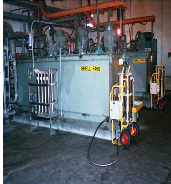
The picture above shows two FM 504's connected to the lube systems and one of the new FM 840 fixed units that have now been installed at Ernest Henry
