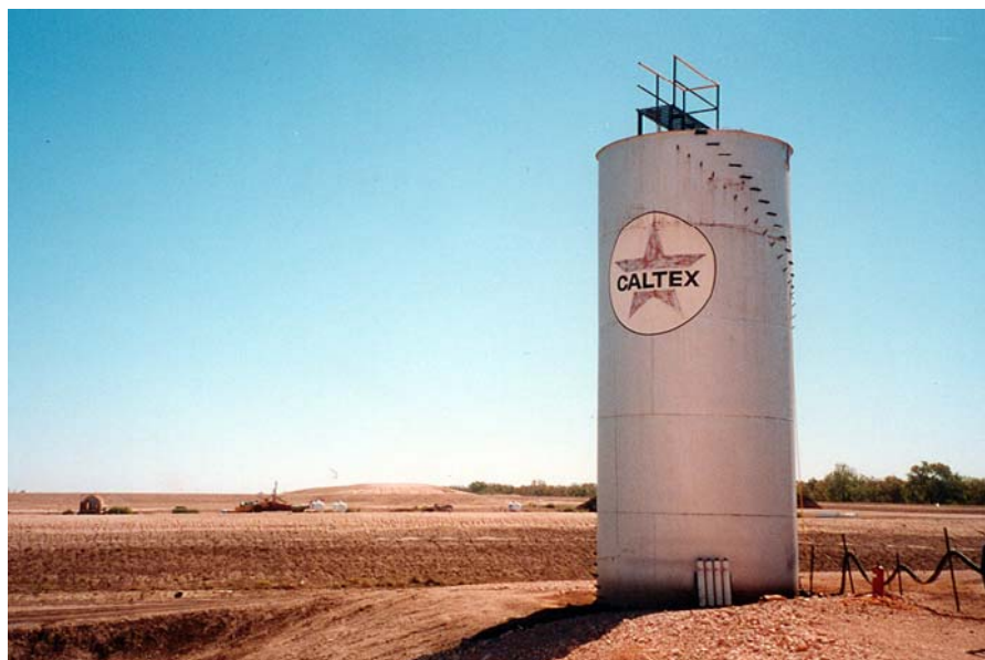
Cubbie Station Fuel Storage Tank
