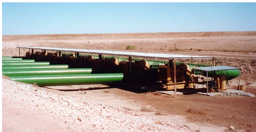
Seven Cat 3406 engines drive water supply pumps for irrigation
